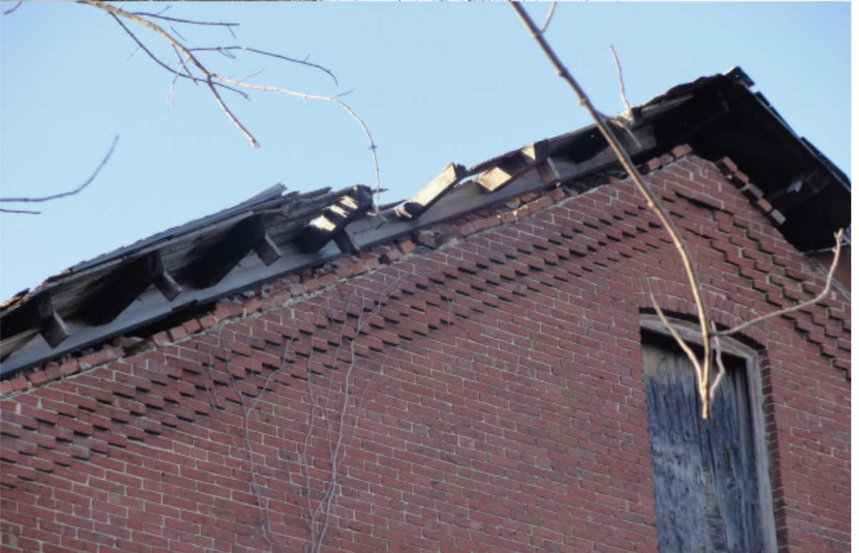
Photo 4. East gable overhang destroyed. [11/2017]
