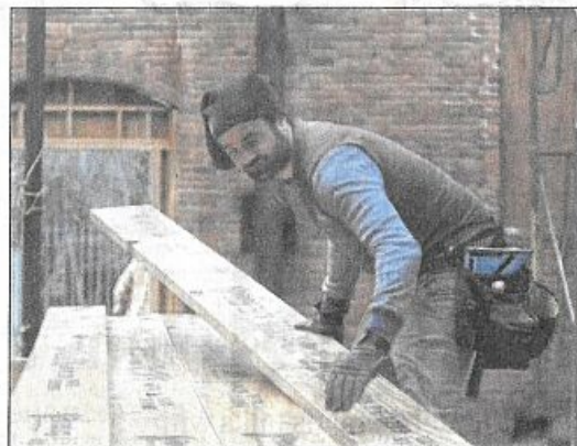
Gabriel Bigger of Worcester stacks rafters that have been measured and cut, ready to use, as he and other workers finish up a day's work on 2 Old Elm St.
